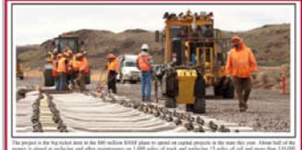
The project is the largest in the history of BNSF. It will include the construction of a new main line that will be 10.5 miles long.
